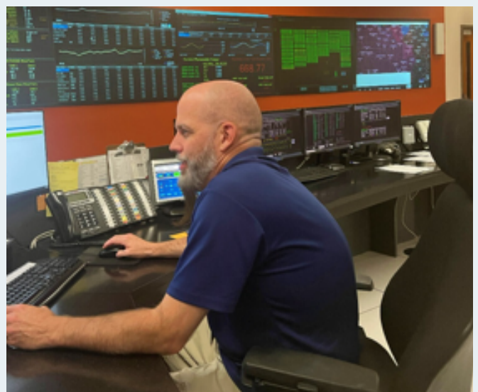
The IMEA state-of-the-art operations center is staffed 24-hours-a-day, 365-days-a-year to serve the needs of member municipalities.
