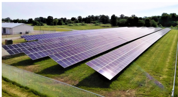
The ½ Megawatt Altamont, Illinois solar energy system became operational in 2020. On behalf of its member municipalities, IMEA commissioned this project through a power purchase agreement with Sol Systems. You can see the live output of this and all of IMEA's solar projects at the IMEA website ( www.imea.org ).
